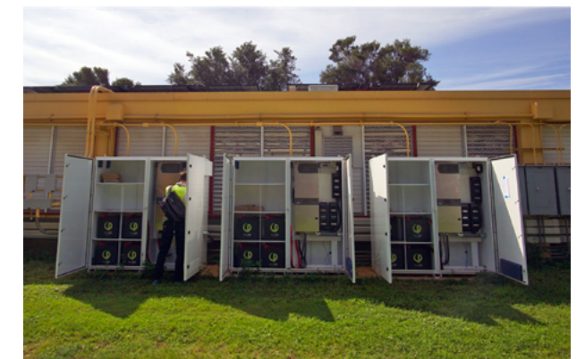
Photovoltaic Air Conditioning System with energy storage
